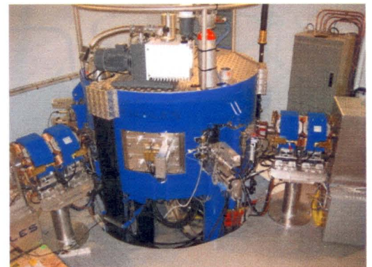
THALES Cyclotron with D-Pace Designed Custom Compact Beamlines, Radiation Shielding, Target Helium Cooling System**, and Load/Unload Process Cabinet with Overpressure**.
